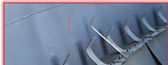
Shunt not making contact with shell.
